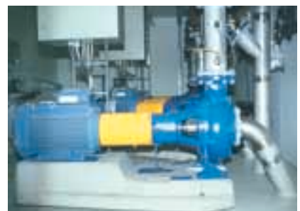
At the waste water plant in Falkenberg, Sweden, FB pumps are handling sewage.
