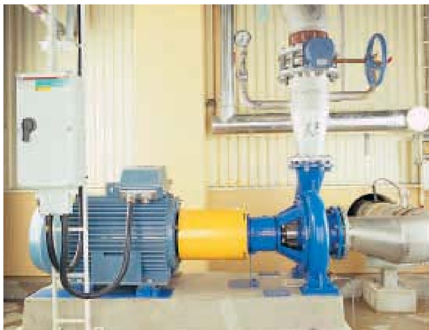
Installation in the chemical industry, Akzo Nobel, Bohus in Sweden. The pump is mounted on a concrete foundation.
