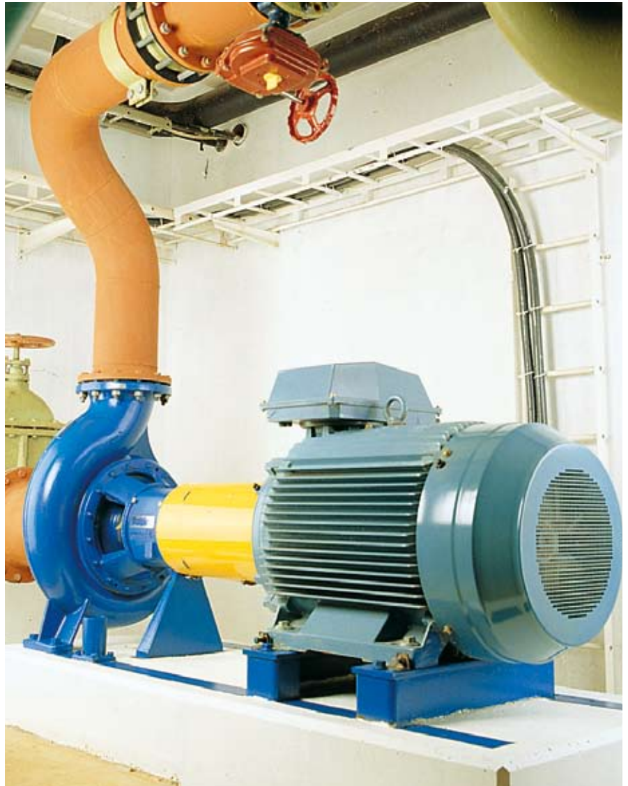
BA 300/250-43 pumping water from Göta river for AKZO NOBEL.
